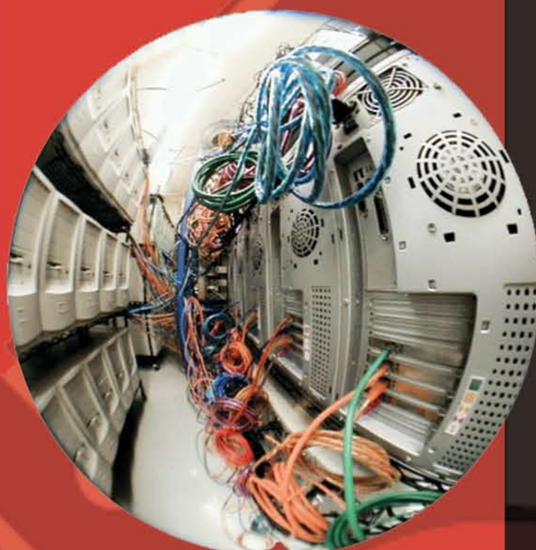
The KLAT2 Cluster Wiring
